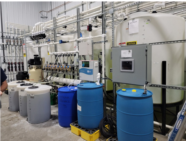
Fertigation room — H.E. Anderson controller and injector bank.
