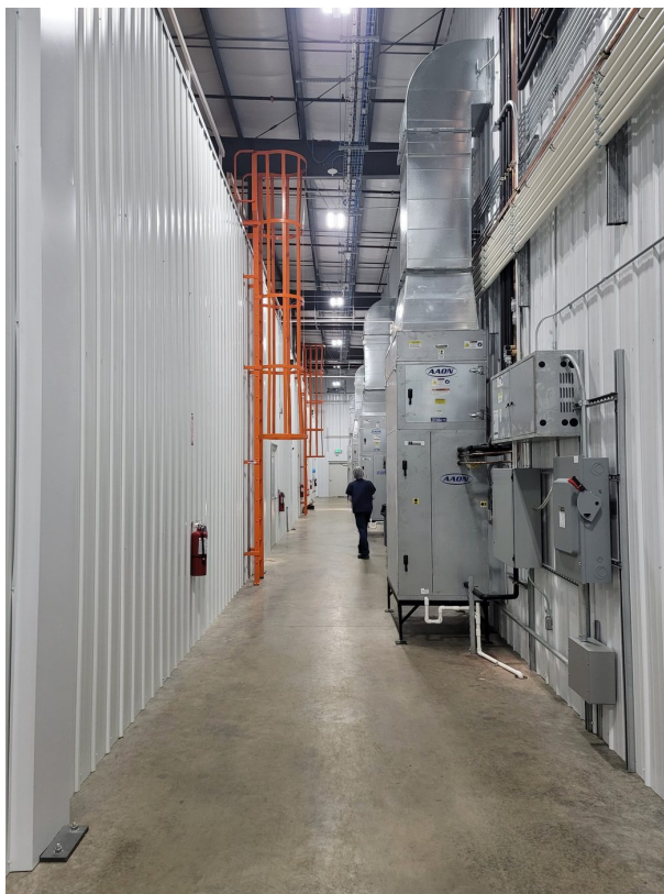
Mechanical corridor — AAON air handlers serving the cultivation rooms.
