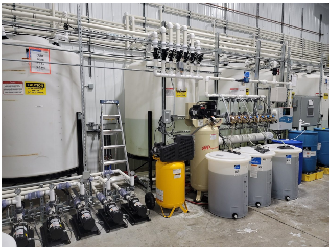
Fertigation room — pump distribution skid and storage tanks.
