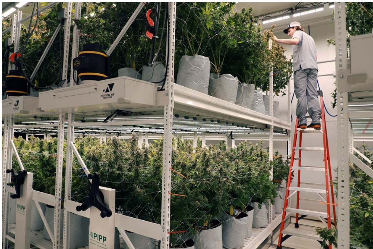
Two-tier flowering room at Redbud Roots, with overhead air-handling units serving the upper canopy.
